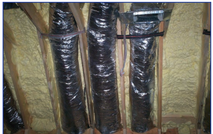
Duct leakage can waste more than 30% of heating and cooling energy. Creating an unvented attic with LD-R-50™ helped contain this leakage within the home to save energy and money.
