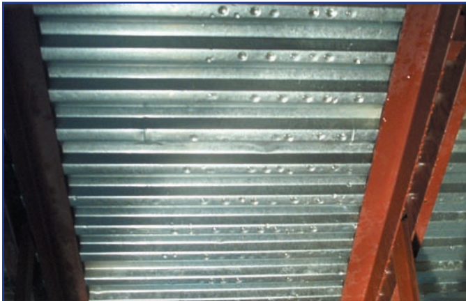
Condensation on the ceiling area below the chillers on the second floor and above the first floor drop ceiling.
