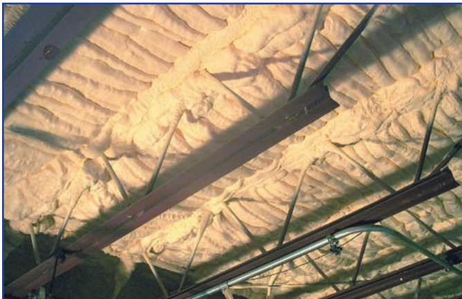
Area of application for Icynene included the footprint of the chillers and walk-in freezers plus a perimeter area extending 10 feet beyond.
