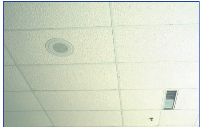
One year after the Icynene insulation had been installed above these ceiling tiles – no more water damage.
