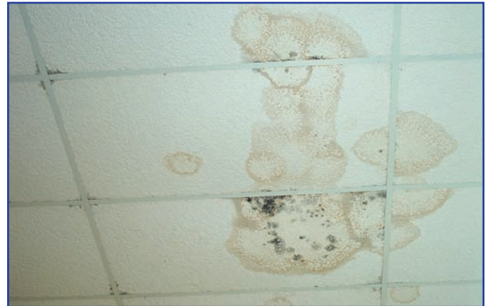
Discolored ceiling tiles were constantly being replaced by Boulineau's who pride themselves on a neat and clean retail environment.
