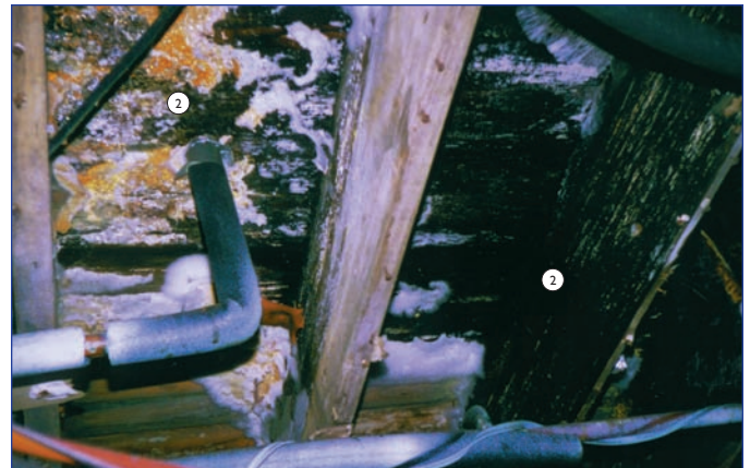
2) Various types of mold and mildew underneath the floors prior to removal and installation of Icnene
