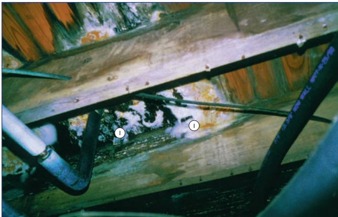
1) Mold problem underneath the floor prior to removal and installation of Icnene
