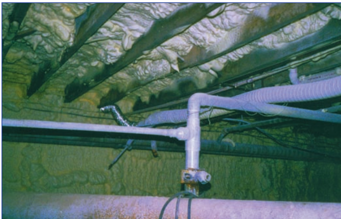
After 3 inches of Icynene was applied underneath the floors and on the walls of the crawlspaces
