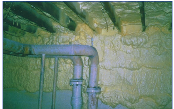
The gaps/cracks were sealed with Icynene to prevent air leakage from the above grade exterior.
