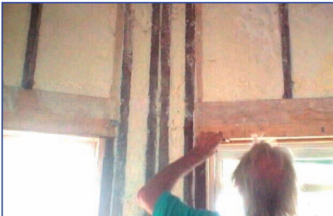
Icynene is sprayed directly into the wall cavity. The foam softly expands to fill all of the cracks and crevices around the studs and window casings. Any excess foam is easily trimmed in preparation for drywall.
