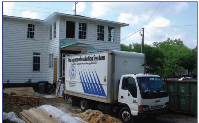
The building had no insulation prior to the renovation. Icyne insulation and air barrier was installed in the walls, floors and attic for reduced air leakage.
