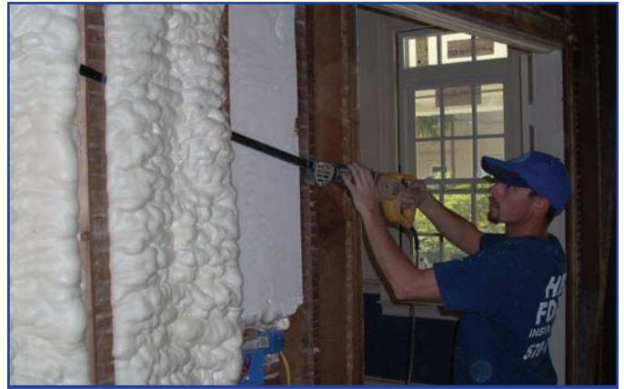
The wall cavities were overfilled and trimmed to ensure a complete fill of insulation in the walls.
