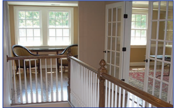
Increased space utilization, improved energy efficiency and reduced energy bills are a few results of this renovation project.
