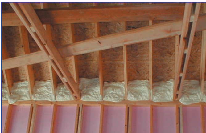
R-18 is sprayed into the rim joists of the basement area to prevent warm, moist air from coming into contact with cooler wall services, minimizing the potential for condensation.
